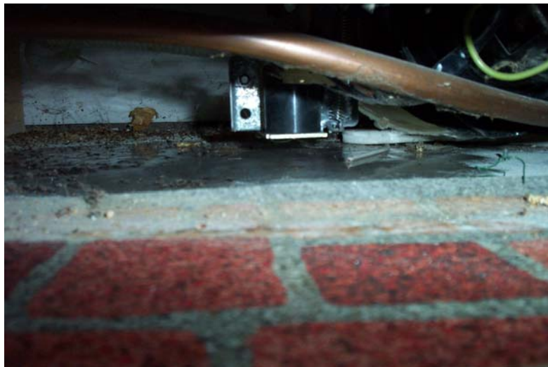
Water leak underneath dishwasher.
