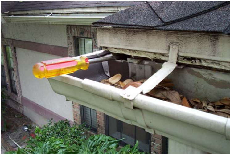
Facia board is rotted behind gutters.
