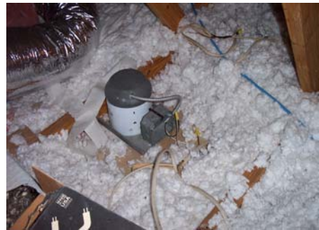
Open electrical wires
