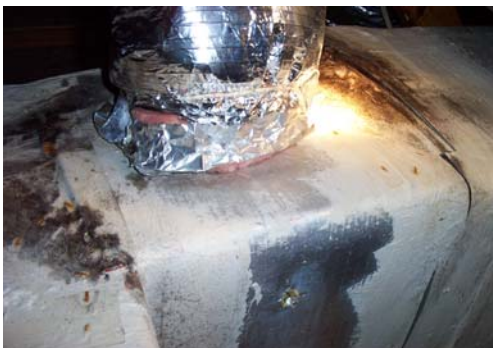
AC duct is not sealed properly
